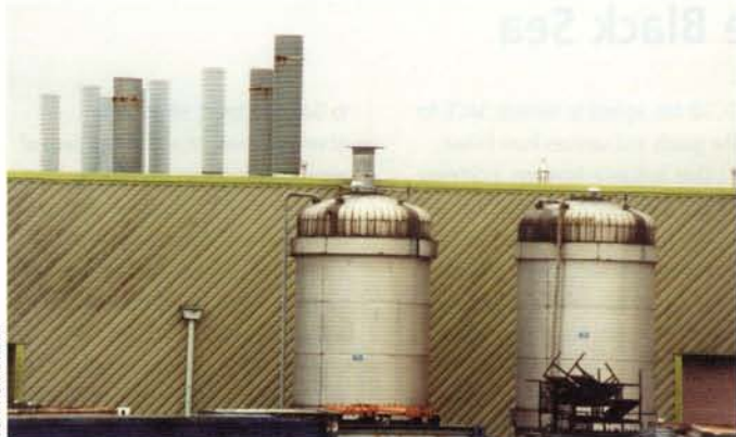
The styrene storage tanks at Ex-Press Plastics' Loddon site. Left are the vent stacks which emit styrene into the atmosphere.
