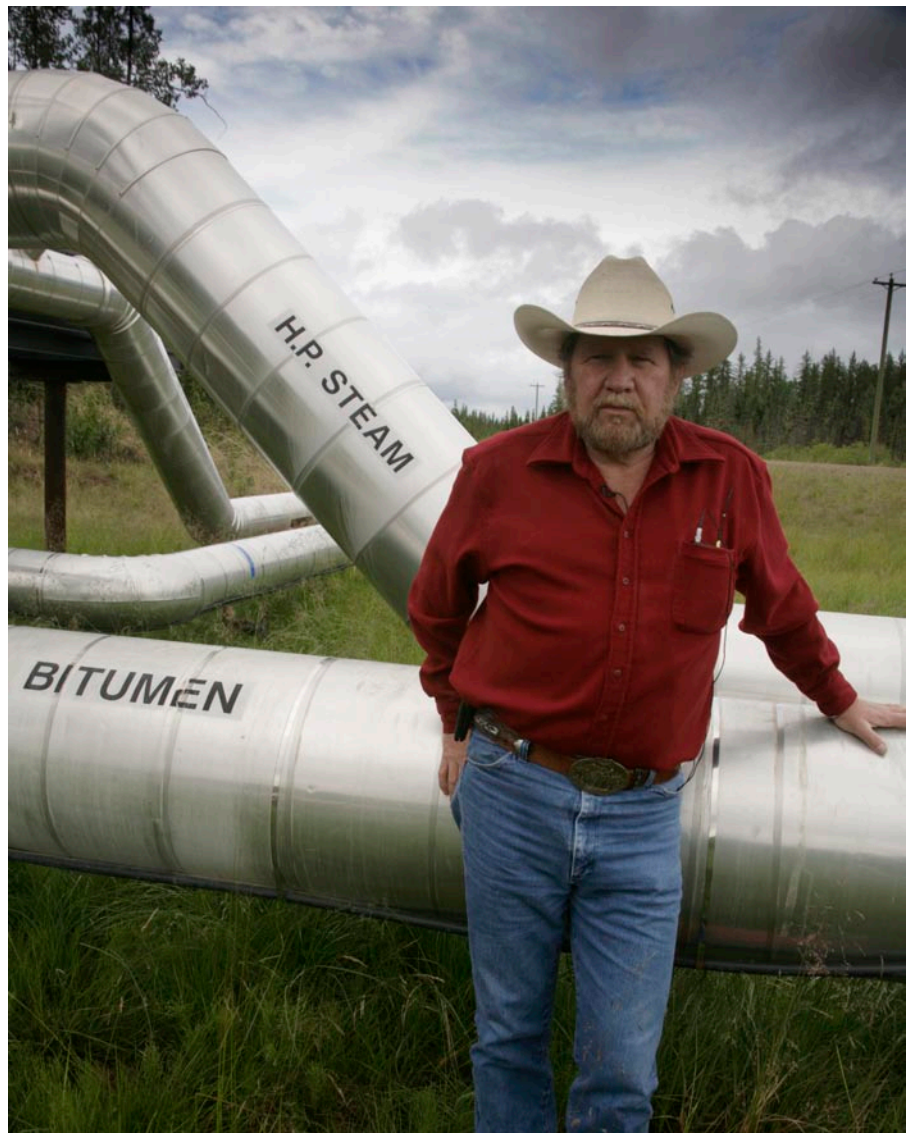
Len Benson stands next to the pipes that supply steam to the bitumen deposits. The Cree believe that the pipes make it difficult for moose and caribou to move freely through the forested area
