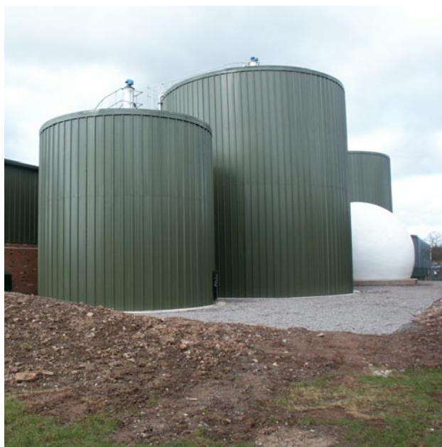
The digestion and gas storage tanks at the Ludlow anaerobic digester. The facility is one of the few operating municipal food waste digesters
