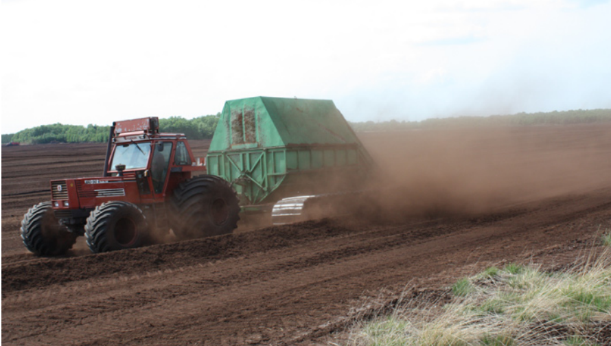
Peat extraction at Chat Moss before the planning permission lapsed (photo courtesy of the Lancashire Wildlife Trust)
