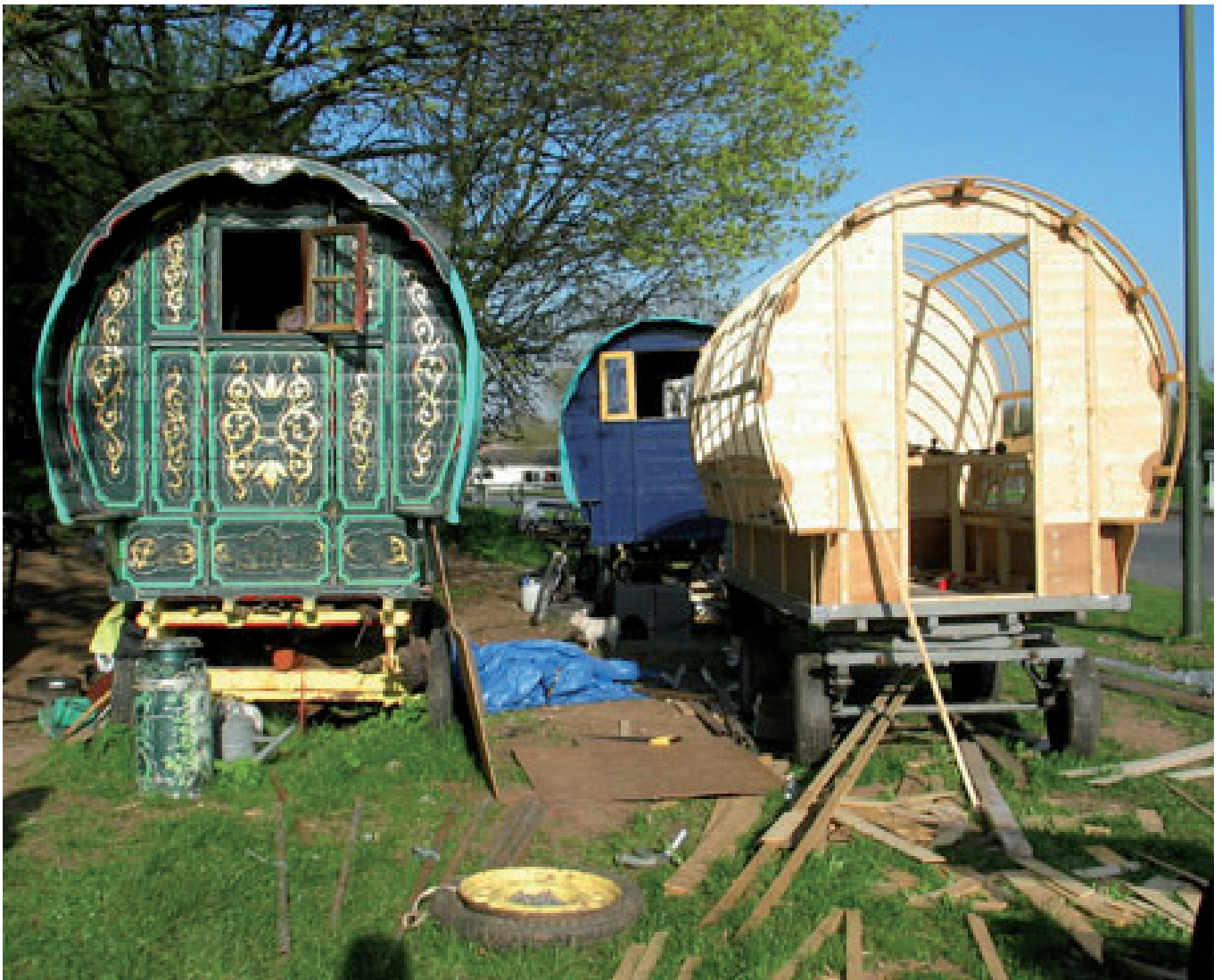
Wagons under construction near Redditch. Unlike many wagon builders, Pete Delaney works where he lives, and has not taken up a yard. Photo: Vjeko Vranic
